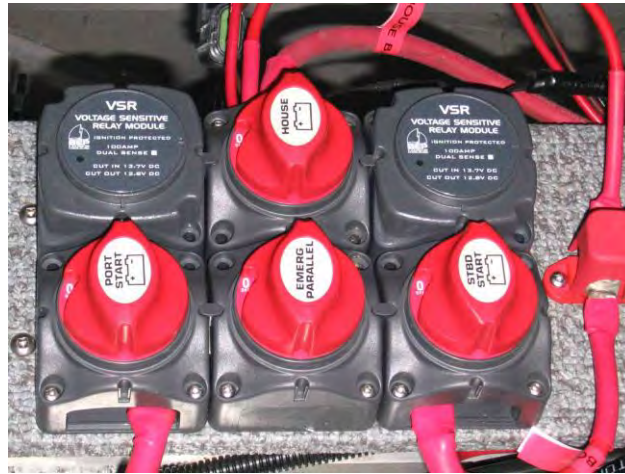
Three bank battery system switches
